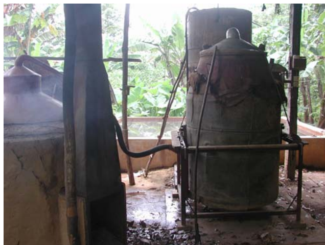
Photo 3 Steam boiler (foreground), still vessel, and fixed pond condenser
